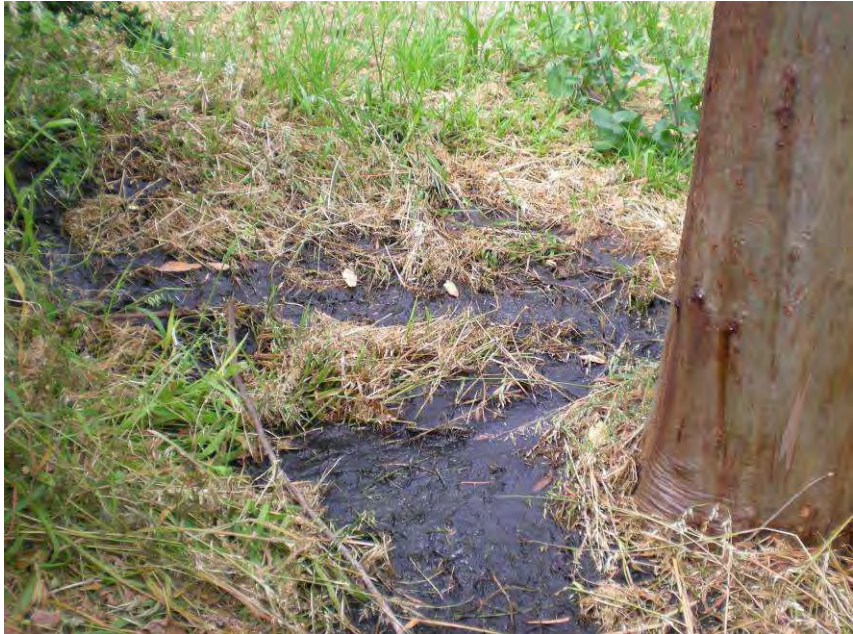
"Overflowing septic tank"
